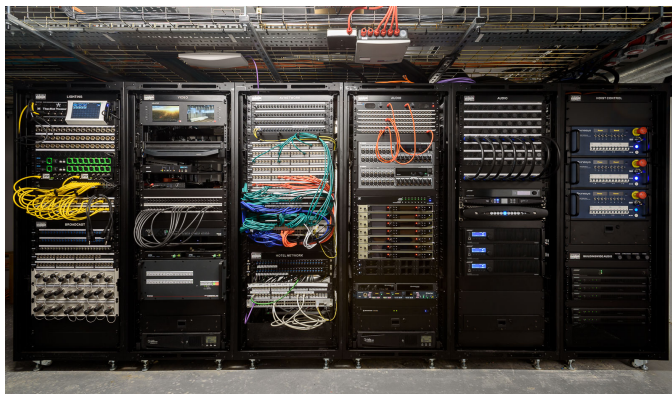
There is also a dedicated broadcast infrastructure with hybrid fibre optical cables at The Londoner
